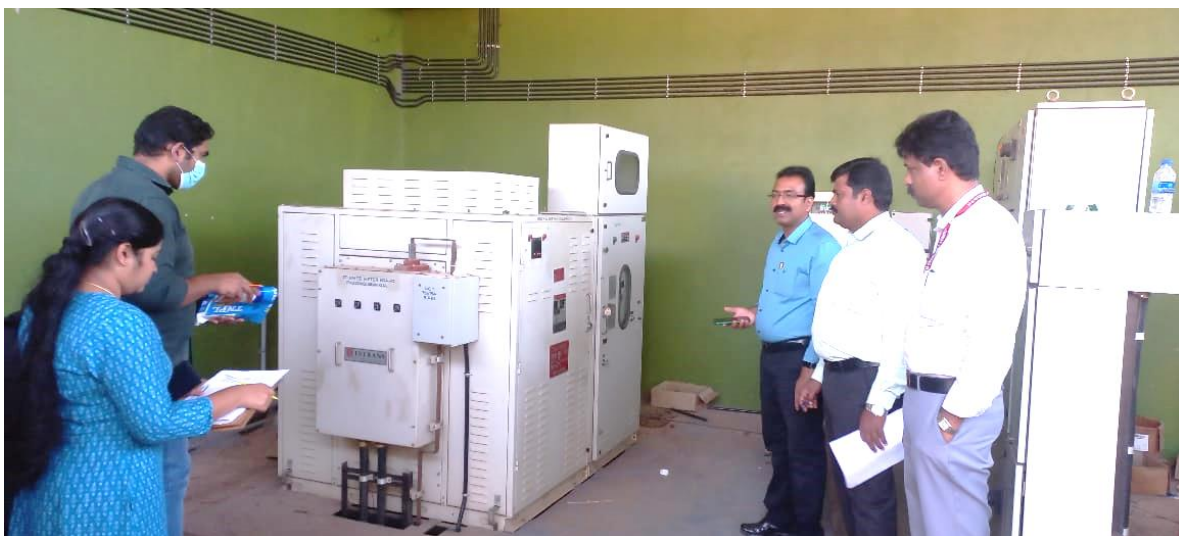
Audit Team members inspecting Energy Devices
